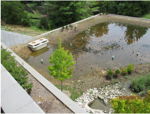
14. All dead grasses in the bio-retention basin need to be replaced.
