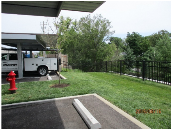
12. The plan shows two trees in this area. Revise the plan to match the site condition for the City's files.
