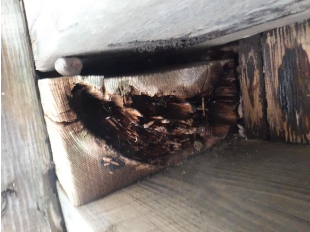
Photo 15 – Existing Timber Approach Span Deterioration
