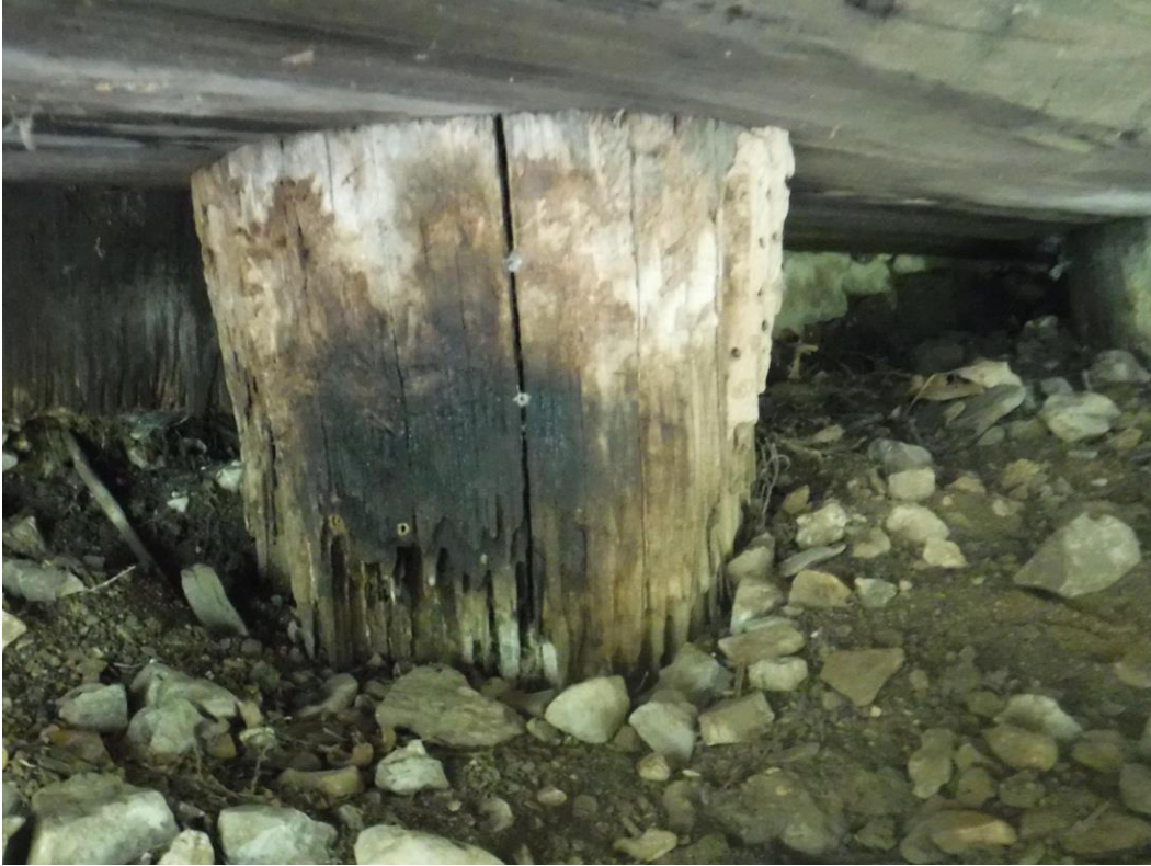
Photo 20 – Existing Abutment Pile Deterioration
