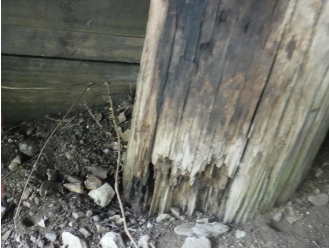
Photo 23 – Existing Abutment Pile Deterioration
