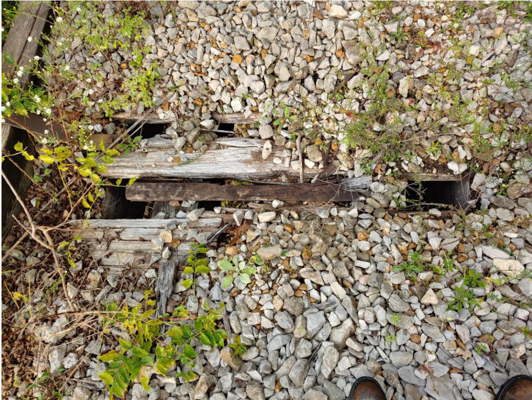
Photo 7 – Existing Ballast Deck Deterioration
