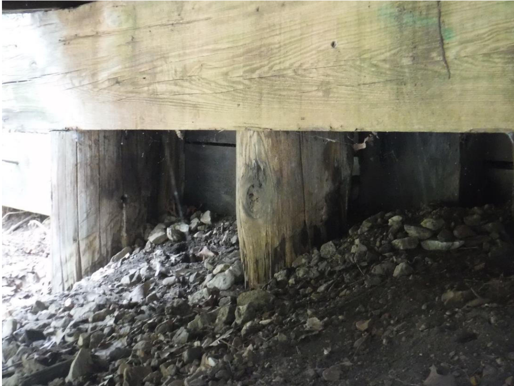
Photo 21 – Existing Abutment Pile Deterioration
