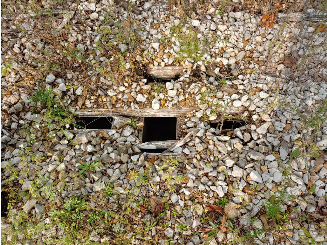
Photo 8 – Existing Ballast Deck Deterioration
