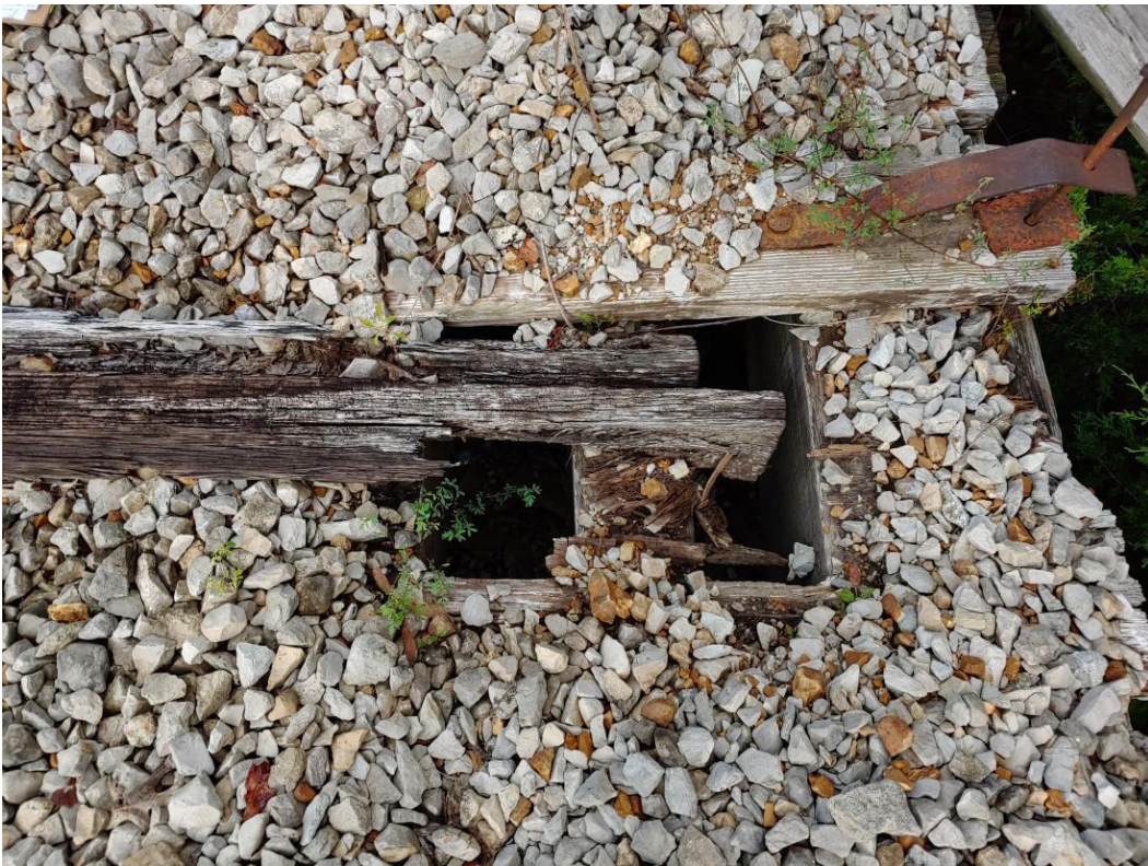
Photo 6 – Existing Ballast Deck Deterioration
