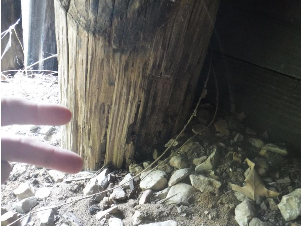
Photo 22 – Existing Abutment Pile Deterioration
