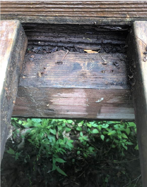
Photo 6 - Typical Exterior Stringer and Main Glulam Decay
