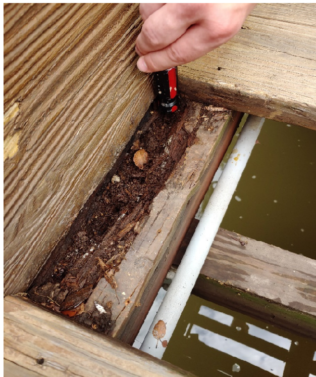
Photo 4 - Typical Exterior Stringer Deterioration
