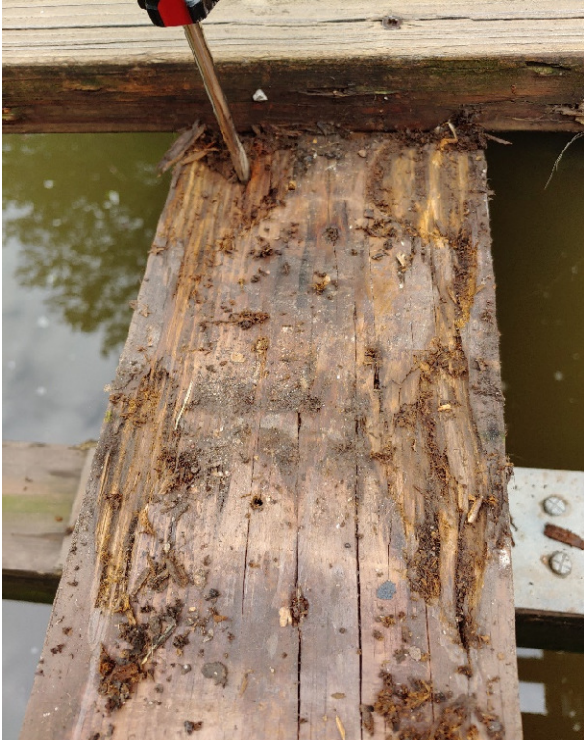
Photo 5 - Typical Interior Stringer Deterioration
