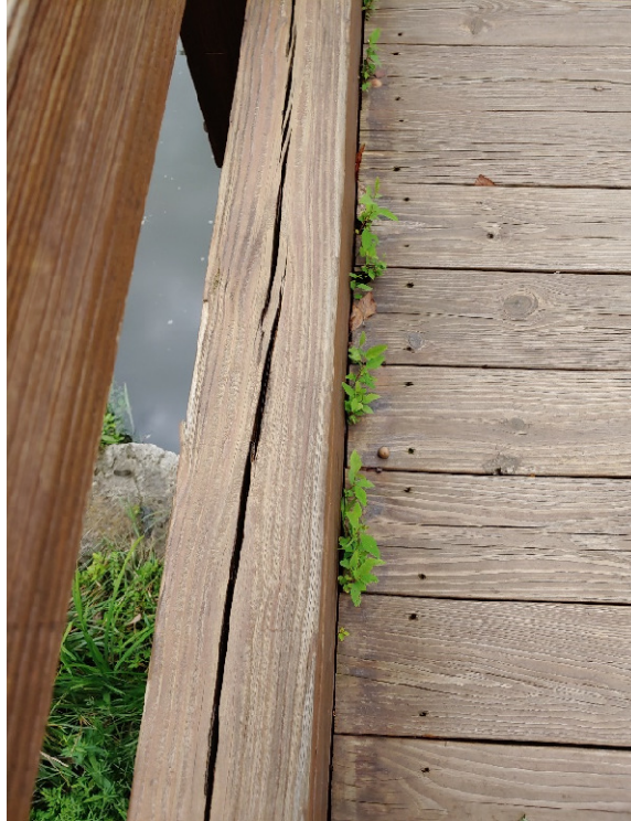
Photo 8 - Large Crack in Main Glulam
