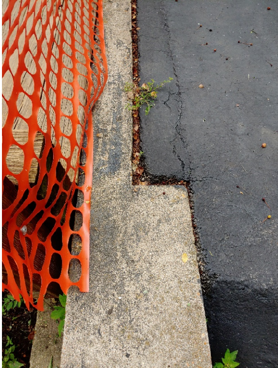
Photo 15 - Approach Pavement Cracking at Joint
