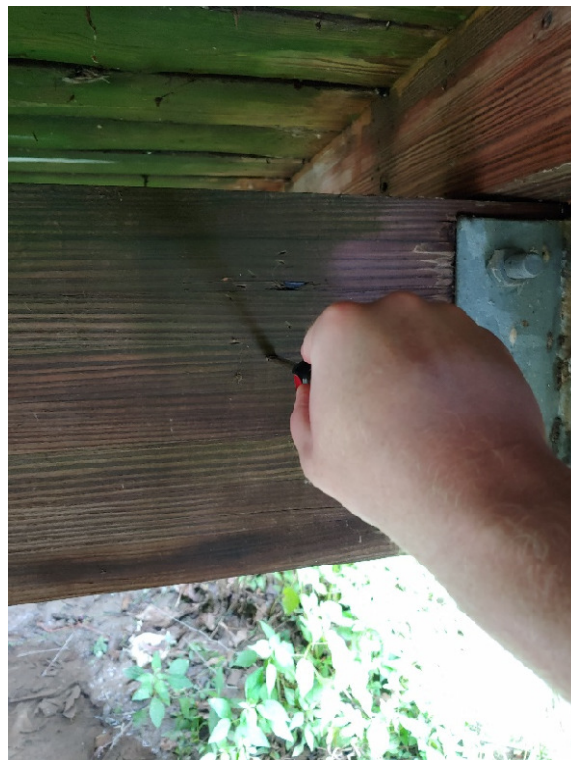
Photo 12 - Floor Beams Soft \frac{1}{8} " into Surface
