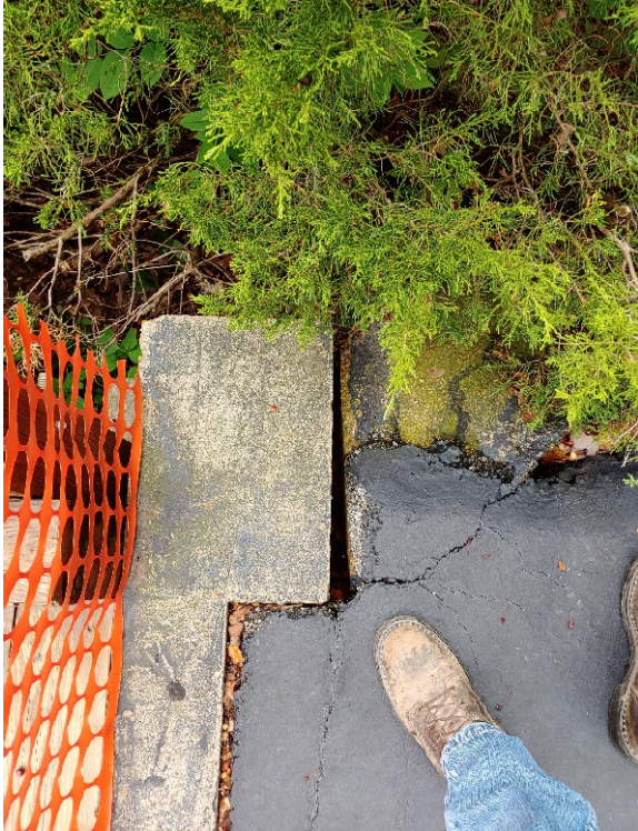
Photo 16 - Detached Piece of Pavement next to West Abutment
