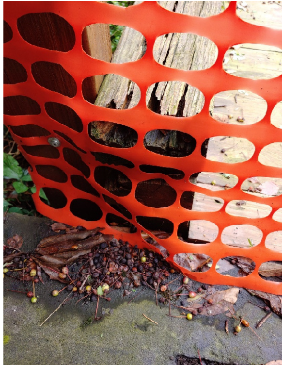
Photo 9 - Section Loss at end of Main Glulam
